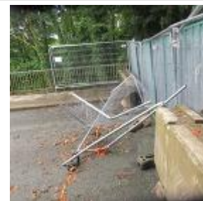
Closure fencing bent and cut needing to be replaced
